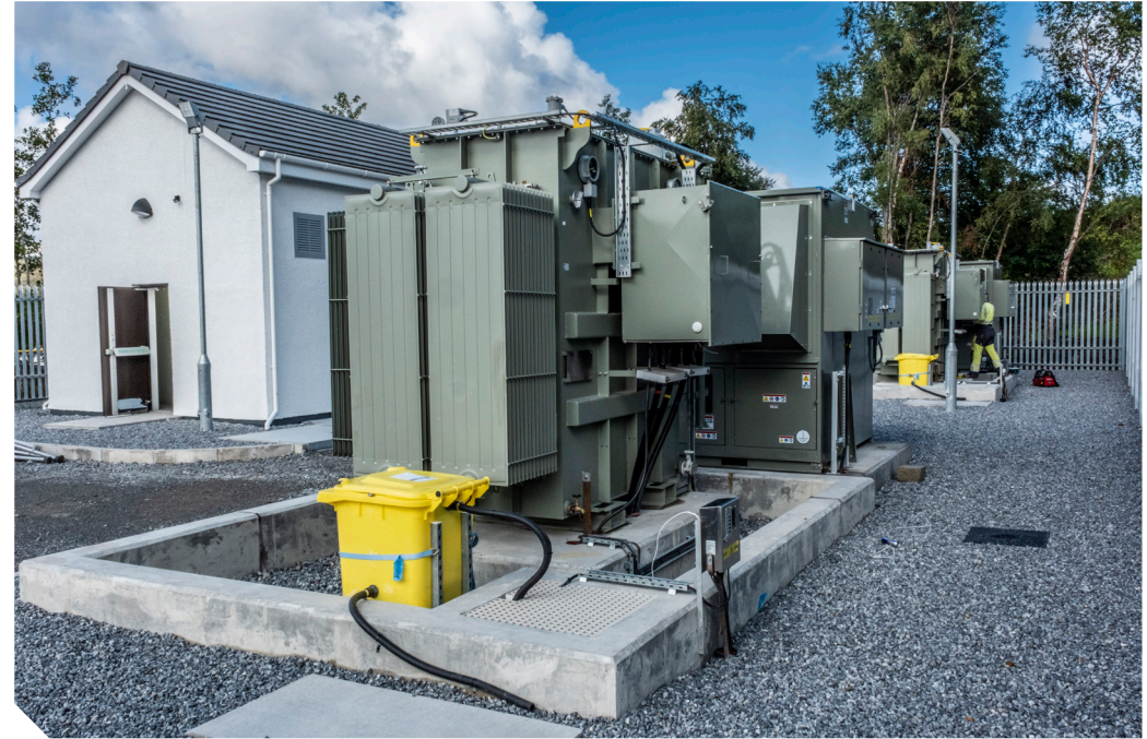
Caption: SSEN Distribution asset
